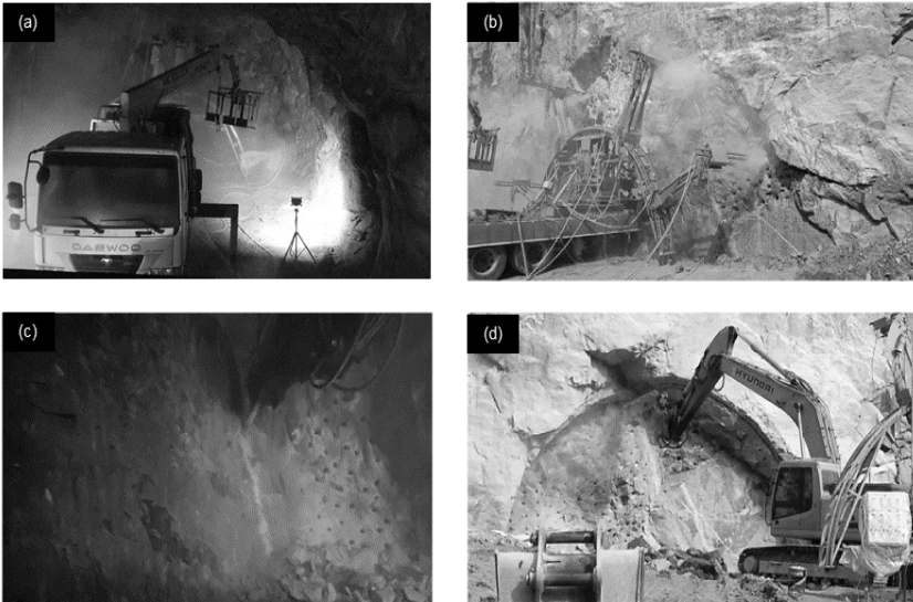
Fig. 7 Abrasive waterjet system combined with hydraulic hammer: (a) Free surface generation inside the tunnel, (b) Free surface generation on the tunnel's portal, (c) Breaking the rock mass inside the tunnel, (d) Breaking the rock mass on the tunnel's portal
