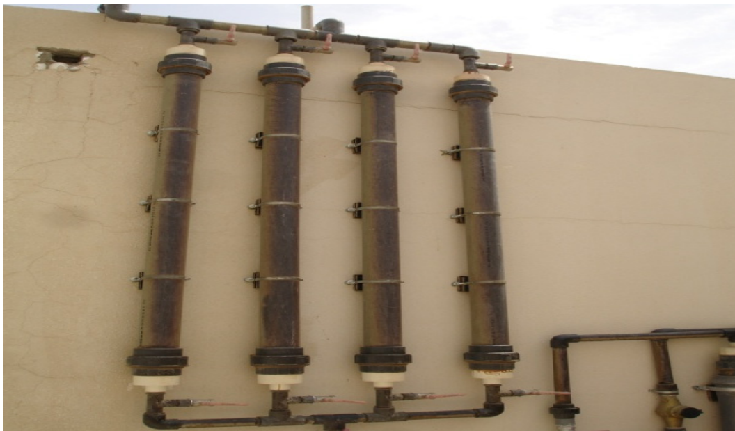
Figure.(2) Sand and activated charcoal filters.
