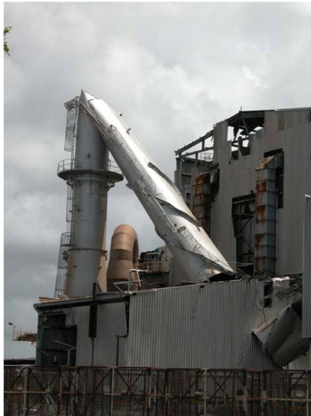
Fig. 9 A failed steel stack equipped with helical strakes
