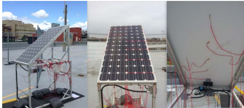
Fig. 1 Site location of PV solar panel: a) Supporting frame, b) Front surface sensors layout, c) Back surface sensors layout
