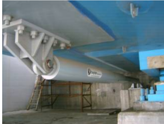
Fig. 10 Longitudinal damper at the girder end of Jiangyin bridge
