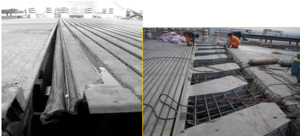
(a) Damage of expansion joints (b) Replacement of expansion joints Fig.1 Damage and replacement of expansion joints for Jiangyin bridge
