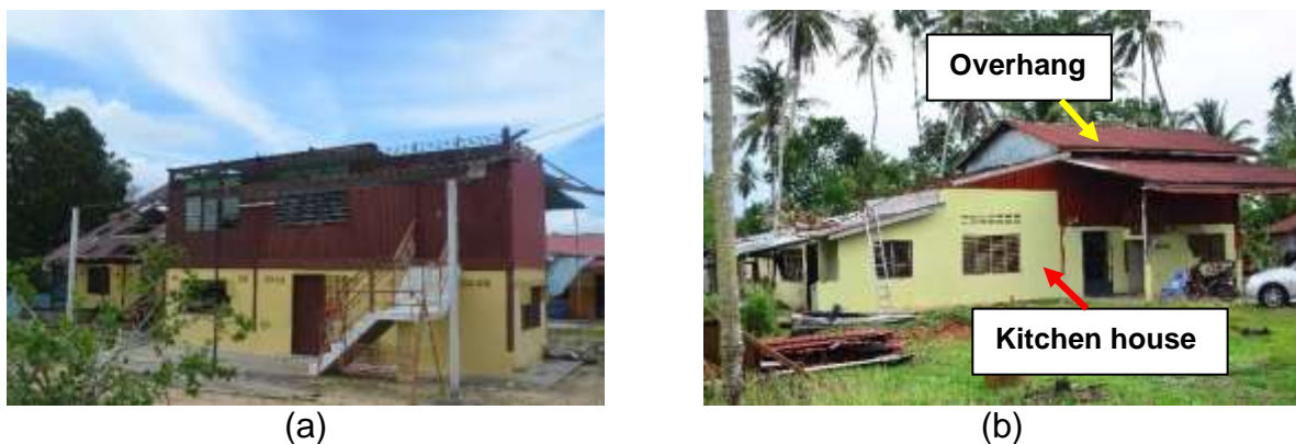
Fig. 1 Damaged to rural houses during windstorm in (a) Balik Pulau, Penang and (b) Kepala Batas, Penang
