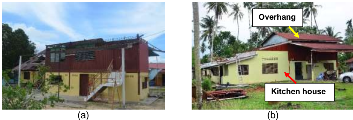
Fig. 1 Damaged to rural houses during windstorm in (a) Balik Pulau, Penang and (b) Kepala Batas, Penang
