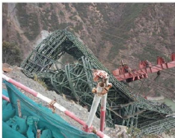
Fig. 1 Collapse of the cable crane during construction of Murong Bridge
