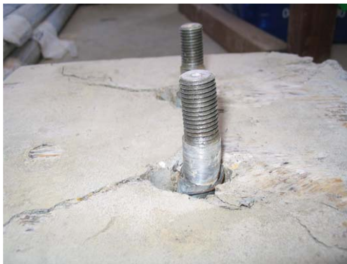
Fig. 5 Concrete crushing – splitting
