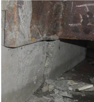
(c). Concrete spalling on the bottom
