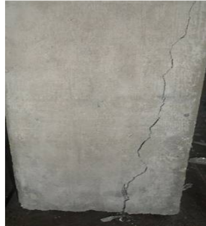
(d). Vertical splitting cracks on the side
