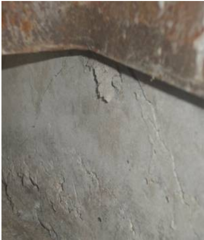
(b). Crack on the bottom
