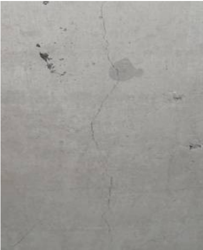
(a) Crack on the side
