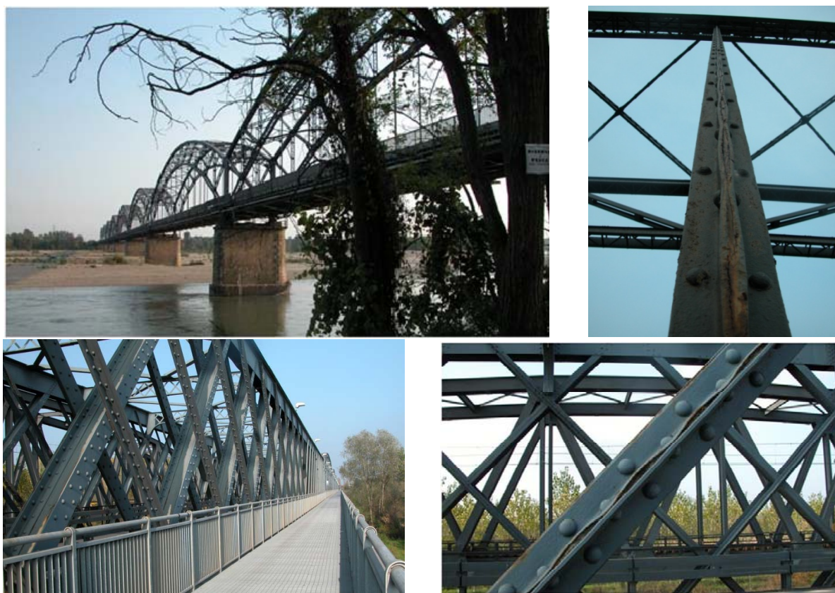
Fig. 1 Truss members deformed by rust swelling
