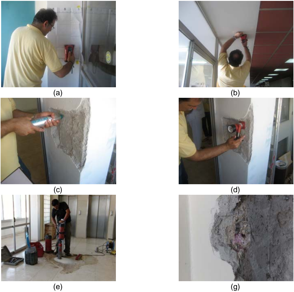
Fig. 3 (a,b) Magnetic tests for detection of steel bar location (c,d) Concrete strength measurement (e) Floor slab coring (g) Detection of concrete carbonation
