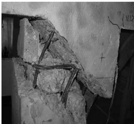
(a) failure of infill
