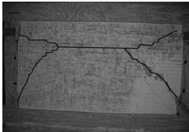
(b) shear failure of frame column
