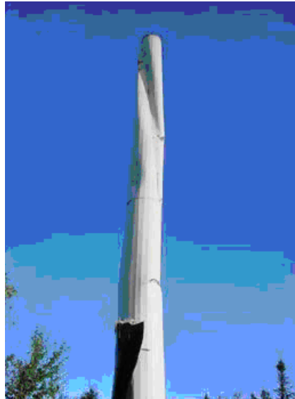
Fig. 1 Torsional Failure of a Wind Energy Tower
