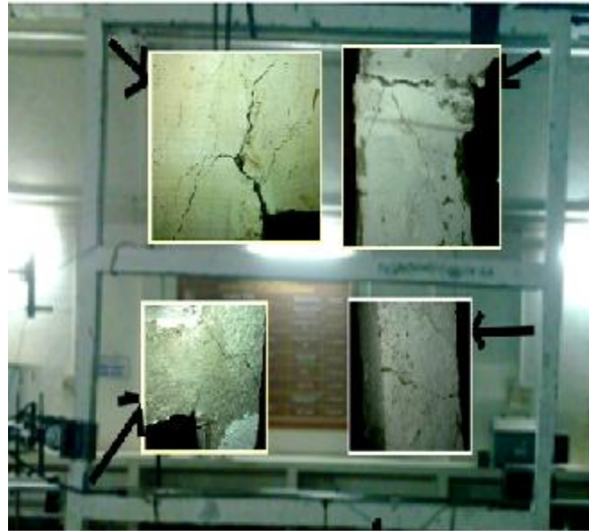
Fig 5. Cracked part of the beam-column joint
