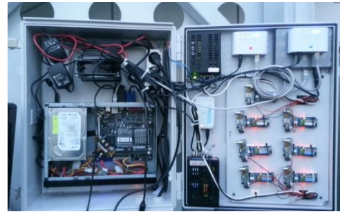
Fig. 5 Experimental setting of data-loggers and storage PC
