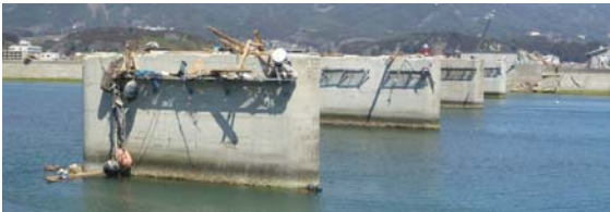
Fig.1 Damaged Situation of Kesen-Bridge
