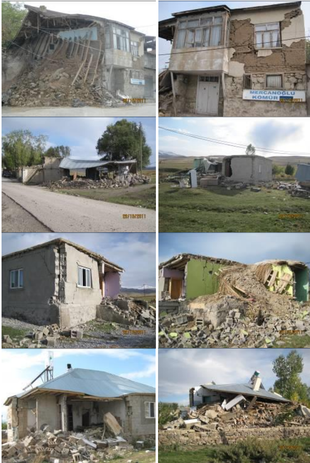
Fig. 1 Common modes of failure of rural masonry structures (Pictures from Van Earthquake -2011-Turkey, Source: Korkmaz S. Z.)
