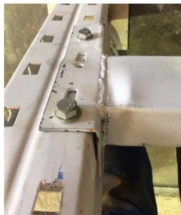
Fig. 7 Failure of bolted beam-to-column connections at beam ends
