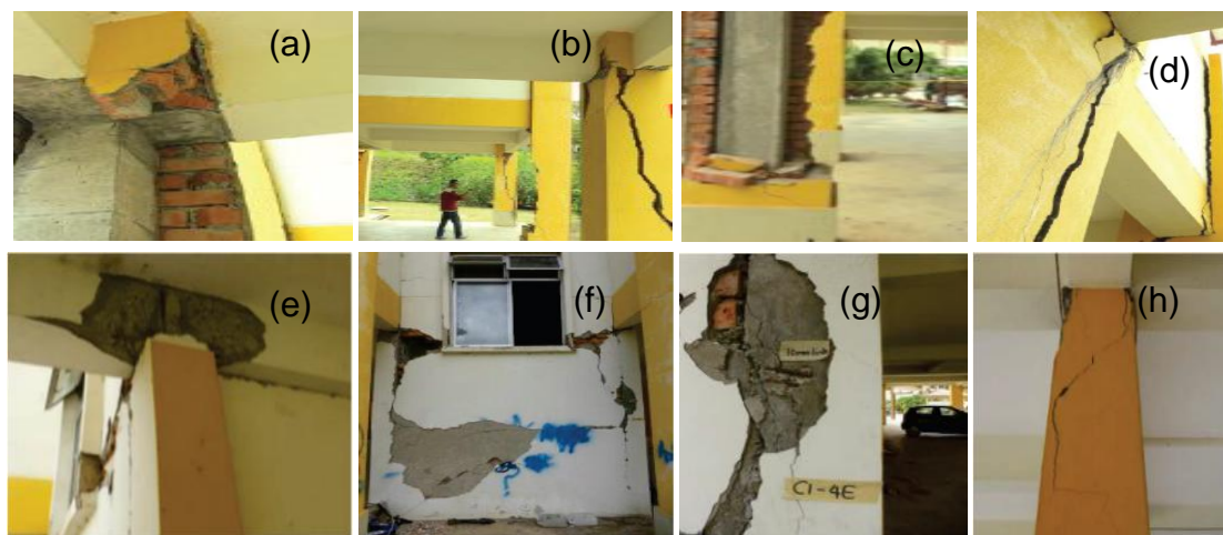
Fig. 4 Observed building damages observed during Ranau earthquake
