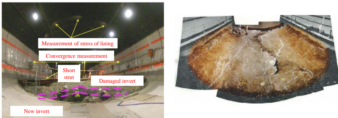
Fig. 2 Example of damage to invert by Heaving (Okui 2009)
