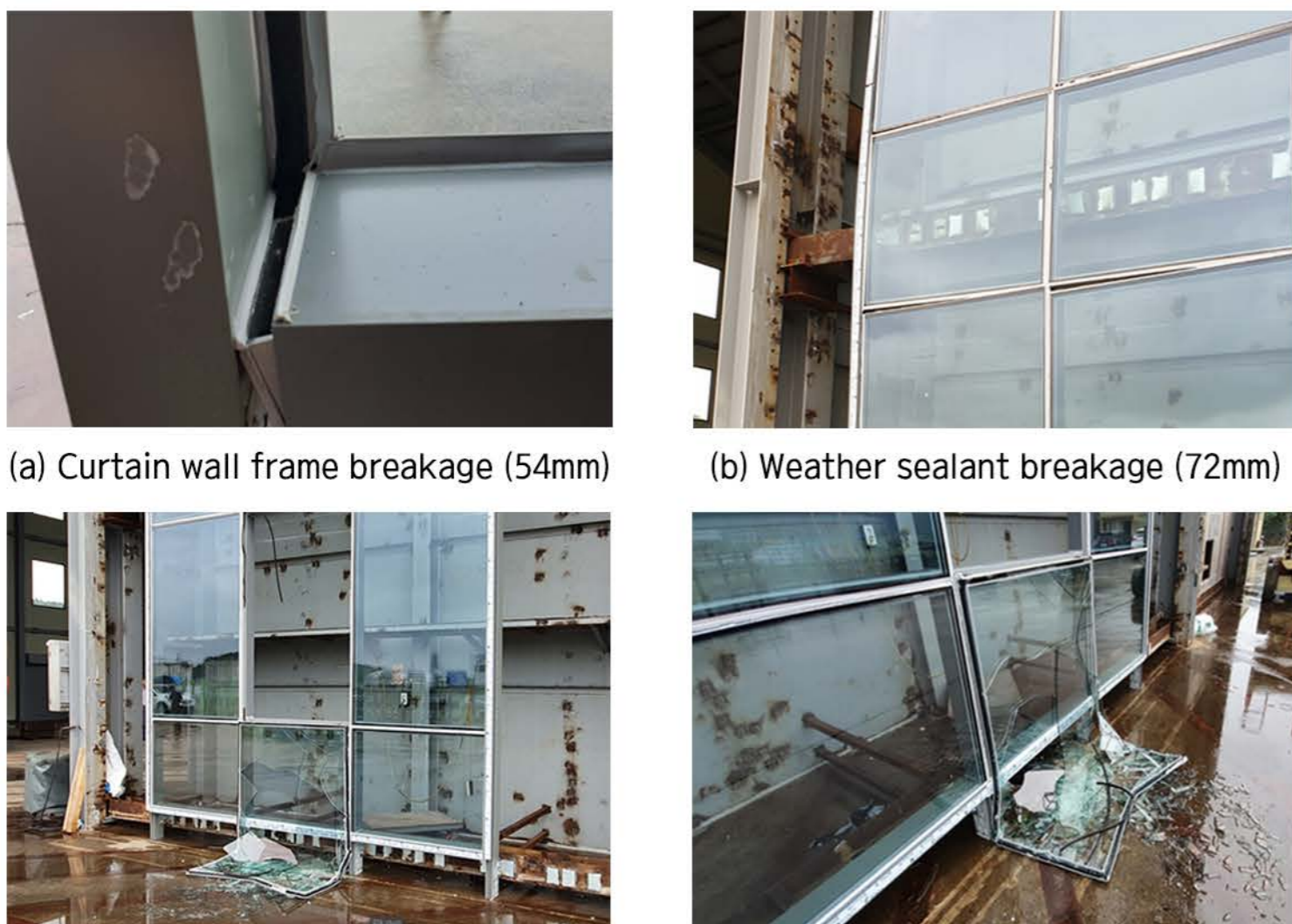
Fig 2. The main vulnerabilities of curtain wall
