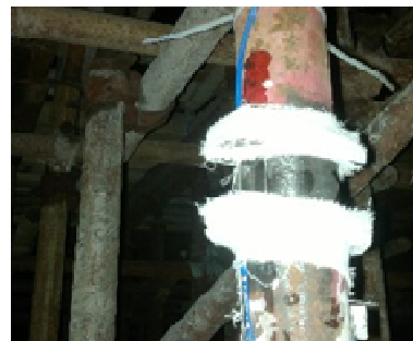
Fig. 4 Protection of FBG sensor in the scaffolding pole
