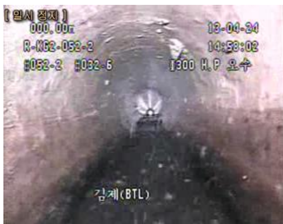
Fig. 1 Sewer CCTV Image
