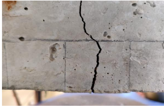
Fig. 5 Crack Pattern in voided beam
