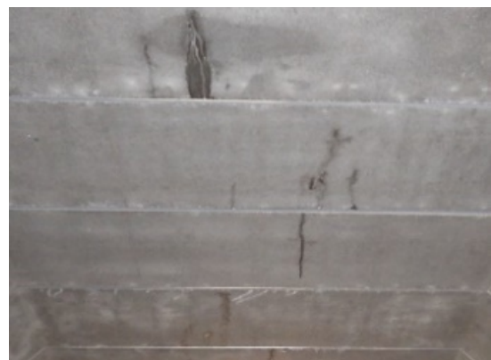
Fig.1 Water leakage from joint gap
